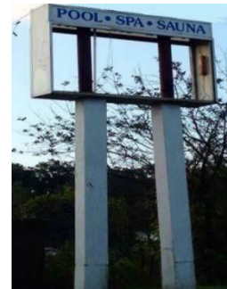
Example of Abandoned Sign
